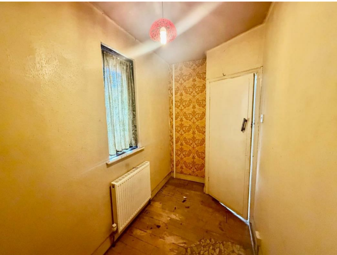
Double glazed window, central heating radiator
