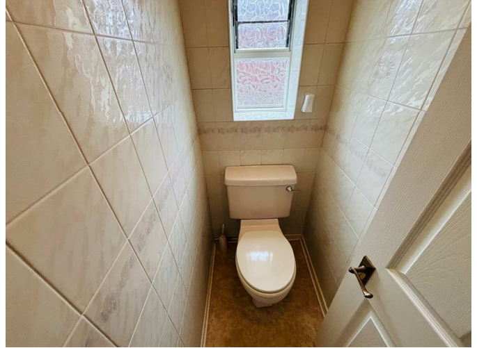
Double glazed window, low flush WC
