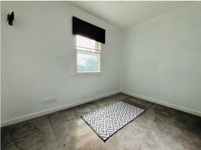
Double glazed window, wall mounted electric heater
